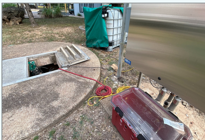
Microbe release tote and oxygenator at a sewer station
